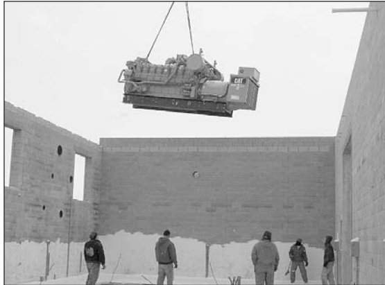
Crews lower the first of four engines to be used to operate the new generation plant at the Jay County Landfill.
